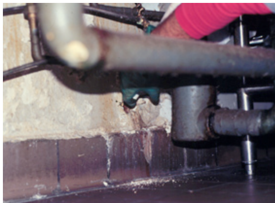
Plumbing leak (Photo by Mike Waldvogel).
